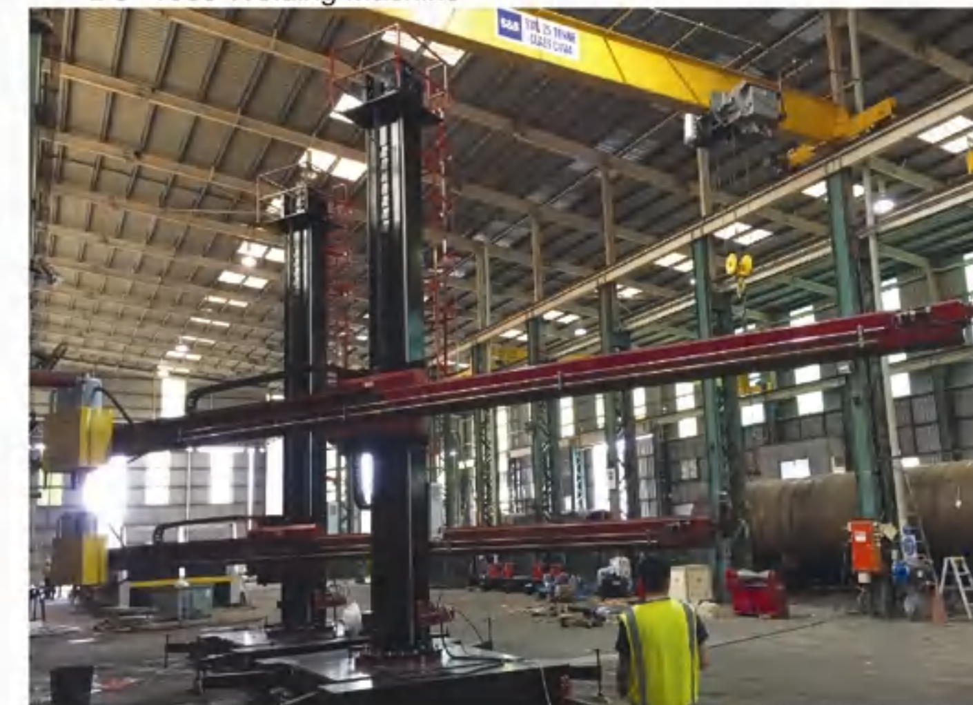
加拿大安装调试5x7焊接操作机配ESAB电焊机 Installation in Canada for 5x7 Welding Manipulator with ESAB LAF1001 Welding Machine
