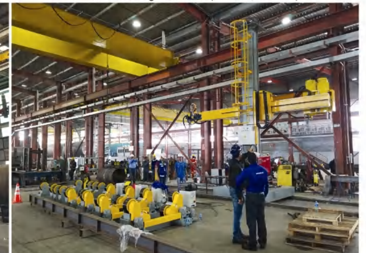
巴拿马安装调试4x4焊接操作机配林肯NA-5控制器 Installation in Panama for 4x4 Welding Manipulator with Lincoln NA-5 Controller
