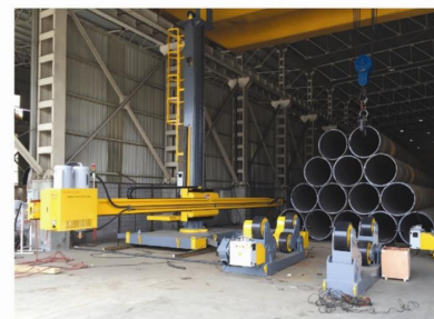
土耳其安装调试5x10焊接操作机 Installation in Turkey for 5x10 Welding Manipulator
